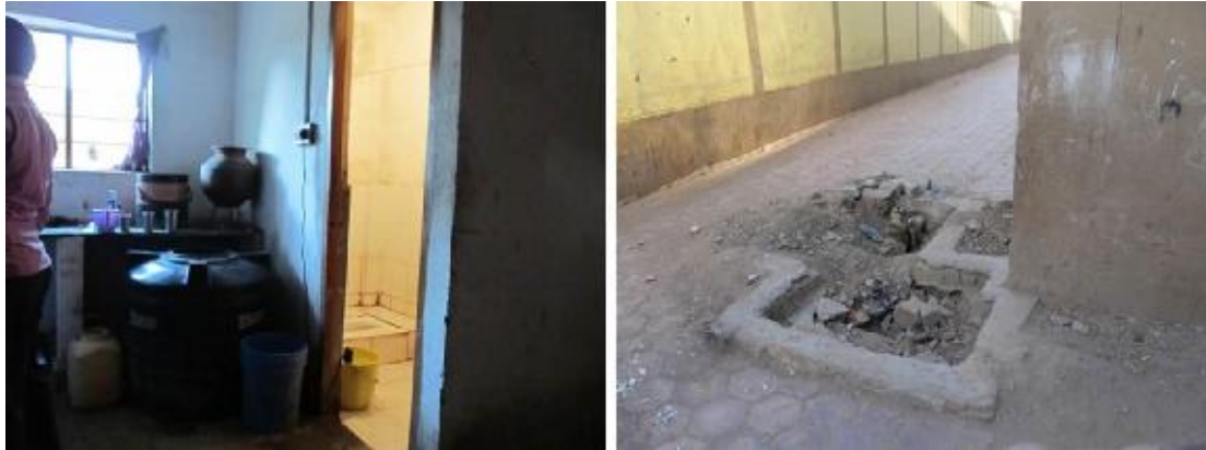
Figure 8: Water tank kept below kitchen platform and entry to toilet from kitchen (left) and dilapidated state of main valve (right)
