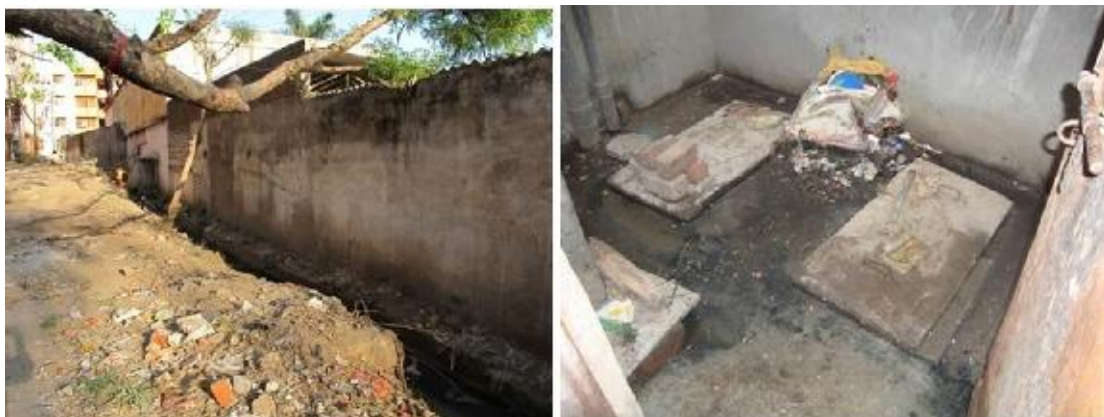
Figure 9: Open drain beside Madrasi Colony (left) and sewage chamber connected to the ground-floor apartment (right)
