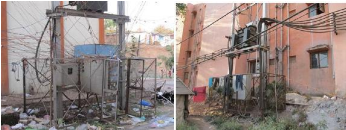
Figure 11: A web of wires in Shabari Nagar (left) and a transformer very close to the window in Madrasi Colony (right)
