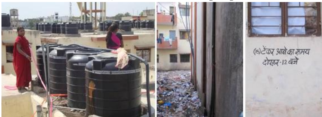
Figure 7: Women filling water from the terrace (left), dangling water mains (middle), and water tanker timings (right)
