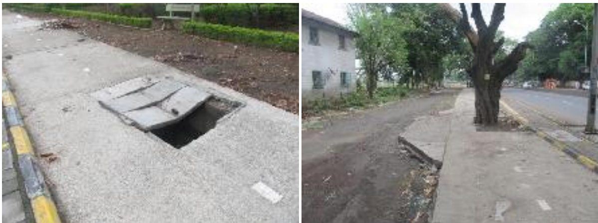
Figure 7: (Left) A Sewage chamber lid left open on a bicycle track (Right) A wedge shaped concrete patch added as afterthought beside a tree.
