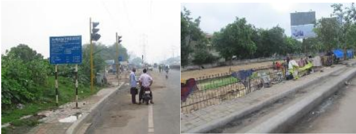
Figure 10 (Left) A JNNURM signboard obstructing the footpath (Right) Unusable width of the footpath and bicycle track
