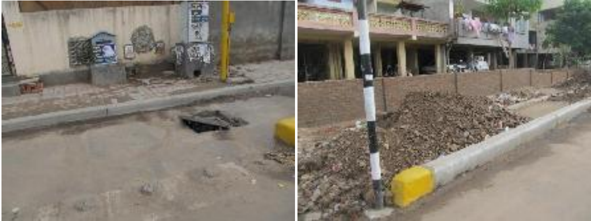
Figure 11 (Left) An open grate on the bicycle track (Right) A heap of construction waste on the bicycle track
