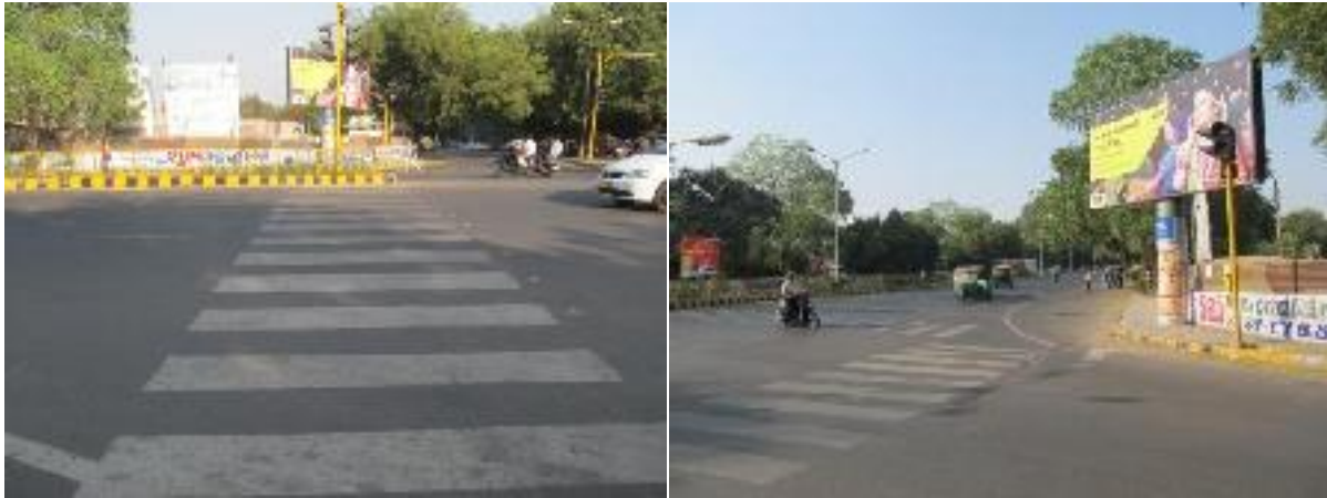
Figure 14: (Left) Zebra crossing ending at a road divider grill (Right) Zebra crossing abruptly ending at turning
