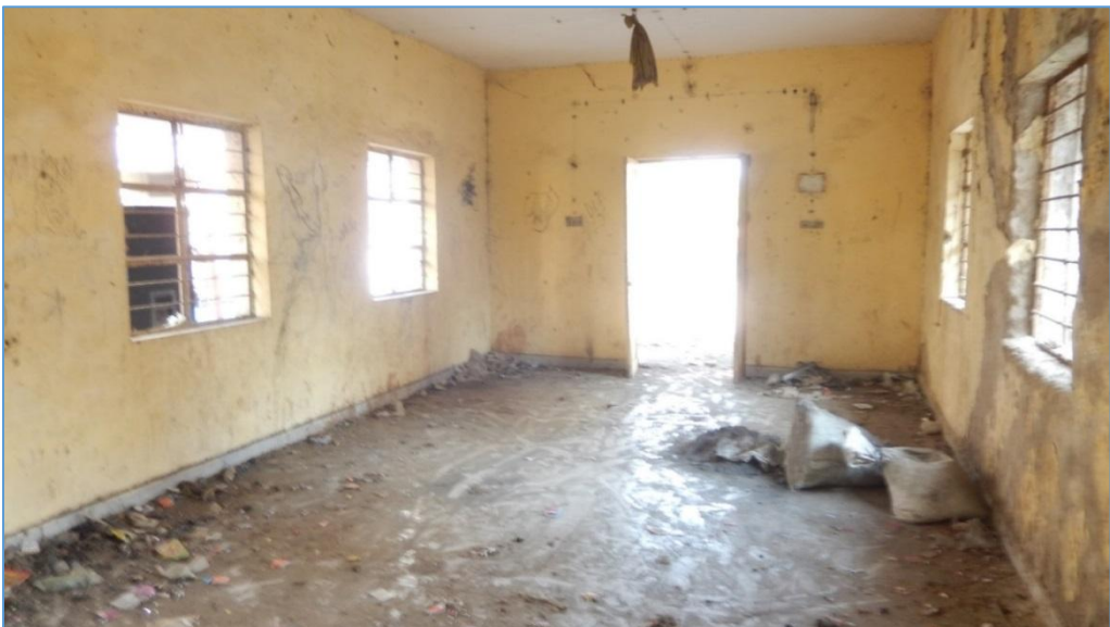
Figure 11: Vacant anganwadi structure at Sundarsinh Bhandari Nagar
